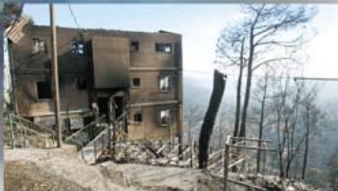
Burned out homes
